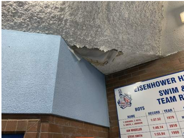
Some issues are easily seen, like the high humidity destroying the ceiling at the City of Yakima Lions Pool. Other issues require a more thorough investigation.
